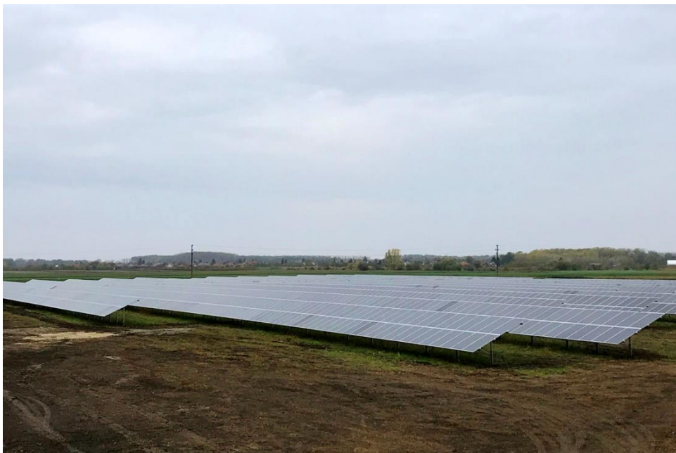
Image by Photon Energy: 1.4 MWp photovoltaic power plant in Kunszentmárton, Hungary.
